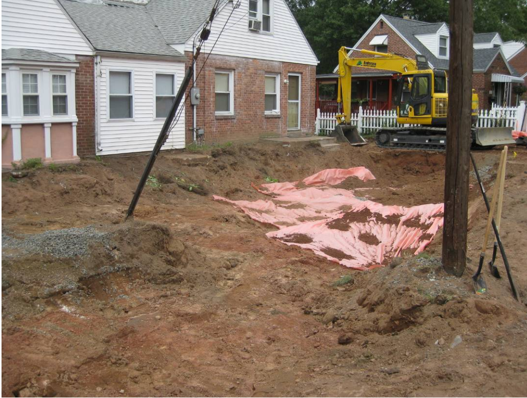
View looking north at excavation in front yard following placement of marker barrier.
