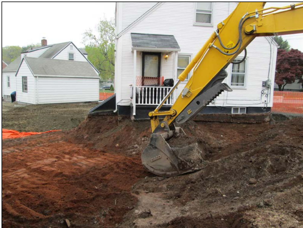
View looking southeast at excavated side yard prior to placement of marker barrier.
