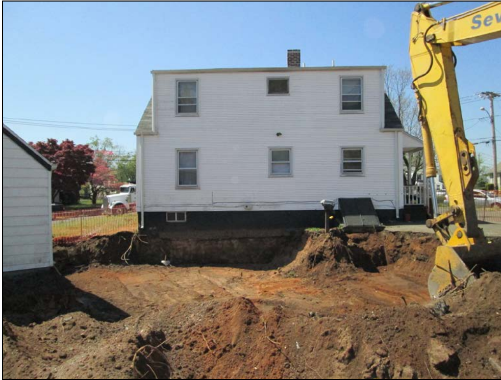
View looking southwest at excavated back yard prior to placement of marker barrier.
