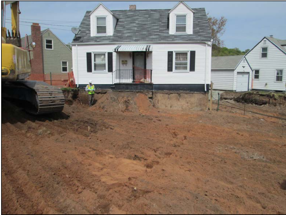
View facing northeast at excavated front yard prior to the placement of marker barrier.
