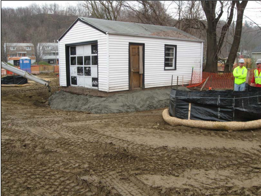
View looking northeast at new drywell and concrete being placed along excavated garage.
