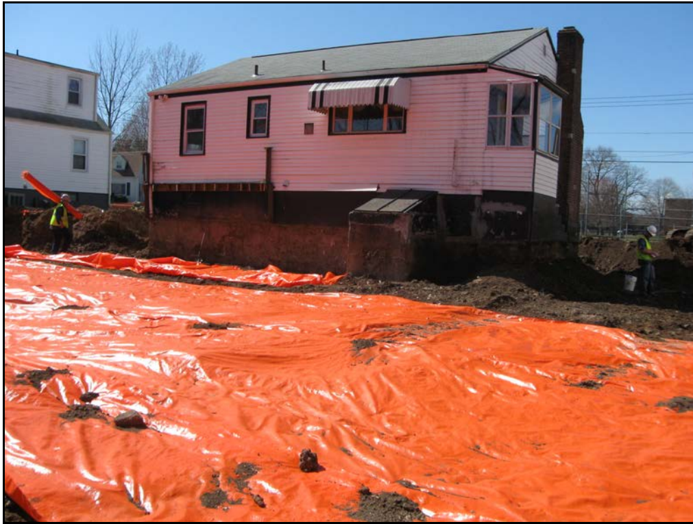
View looking west at marker barrier at the base of excavation of back yard.
