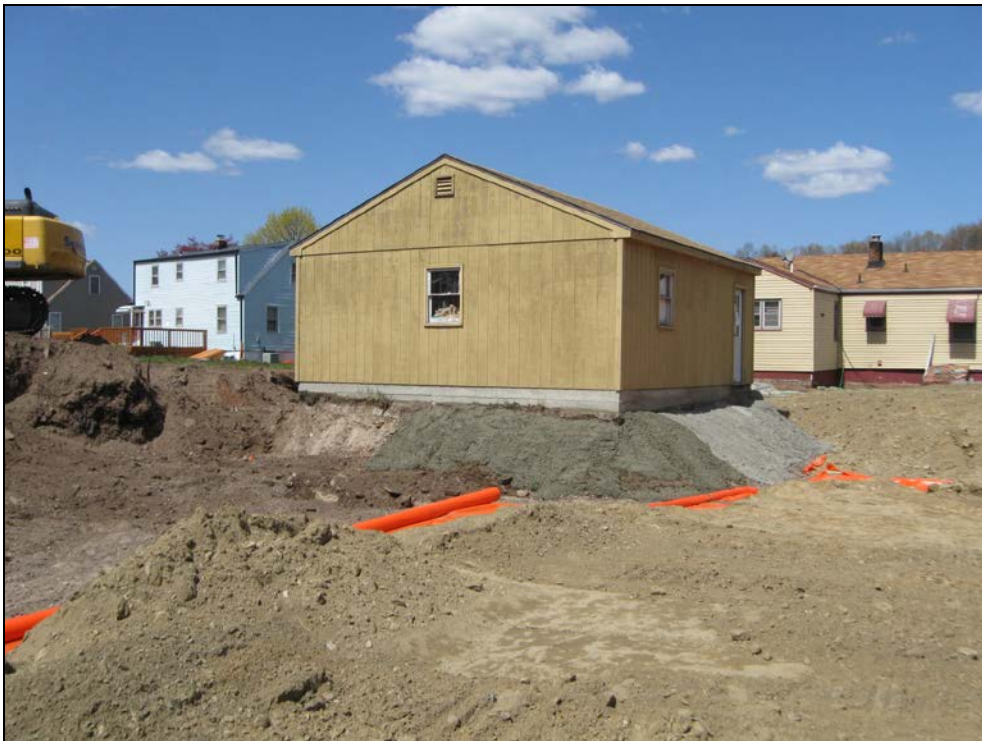
View looking north at excavated back yard with marker barrier over remaining fill.
