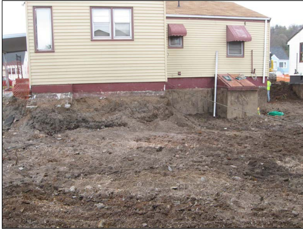
View looking north at excavated back yard prior to marker barrier being installed.
