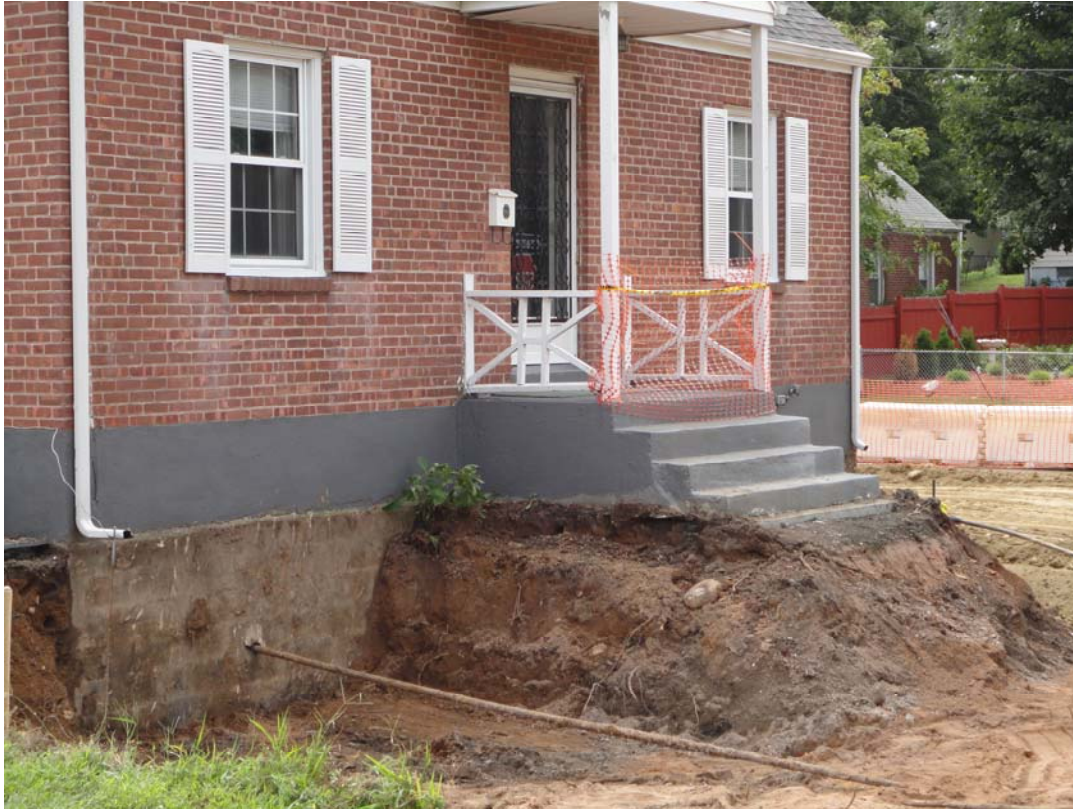
View looking southwest from driveway showing fill remaining around front steps facing Morse Street.
