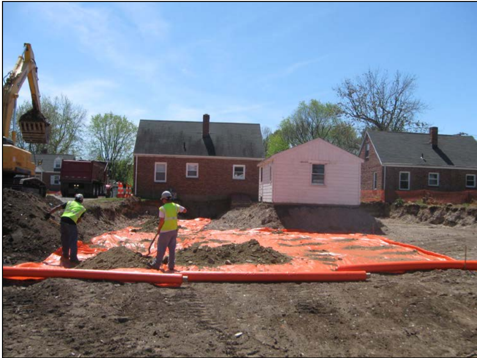
View facing south at marker barrier being installed in the back yard.
