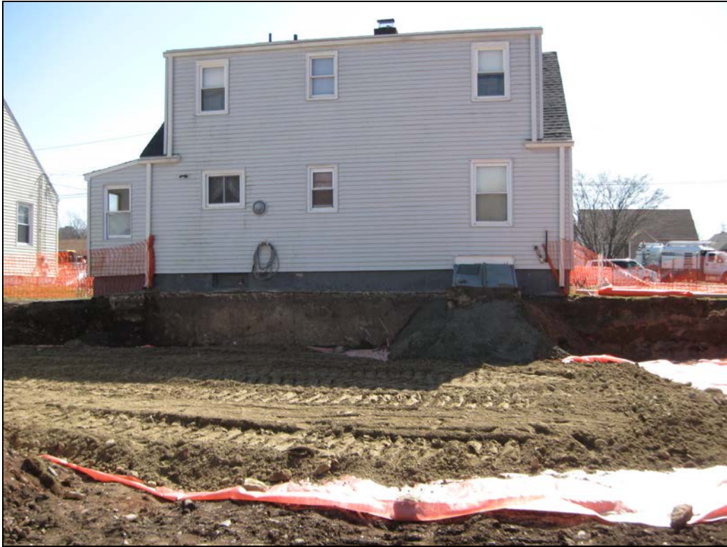
View looking south at marker barrier and concrete in the excavated back yard.
