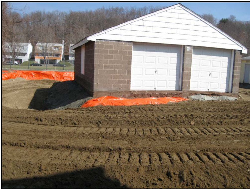
View looking north at partially backfilled back yard showing concrete and marker barrier.
