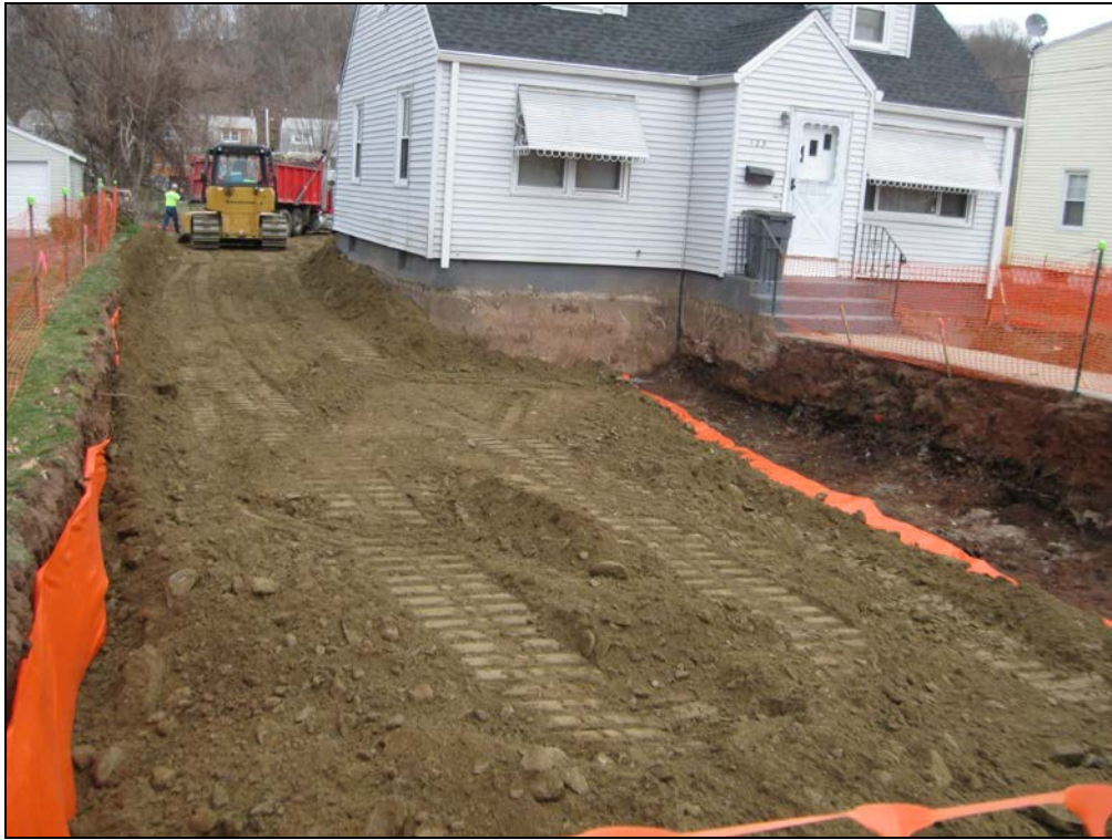
View looking northeast at placement of backfill material in front yard following placement of orange marker barrier.
