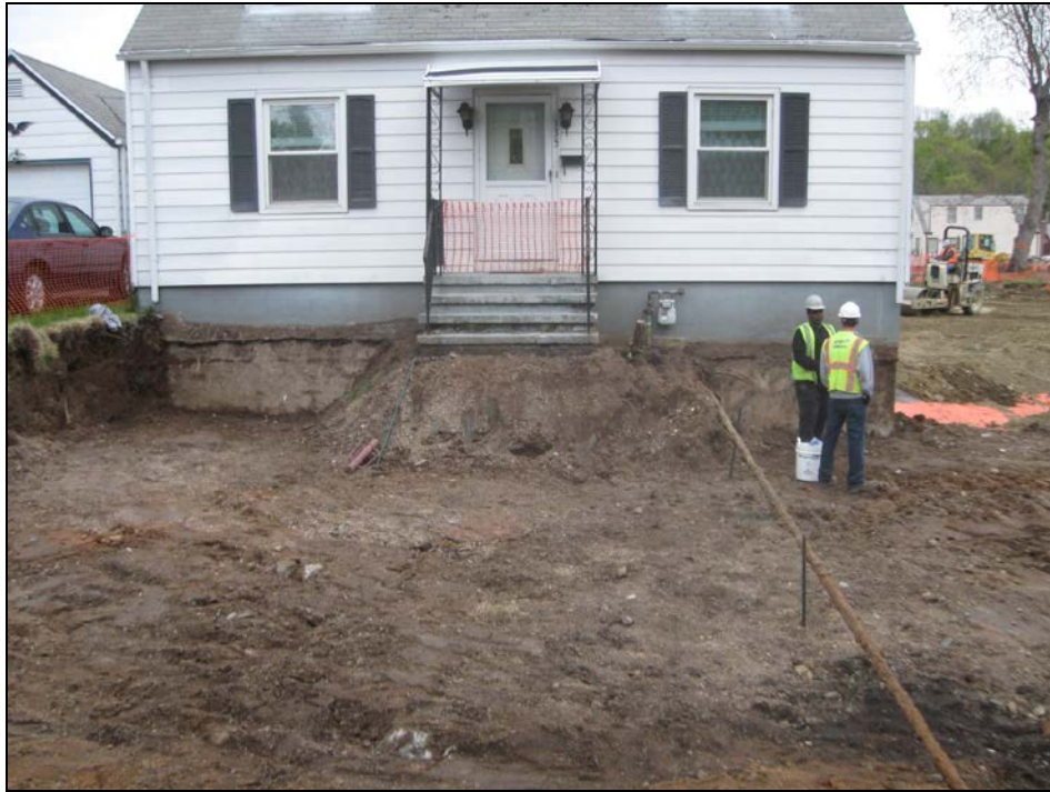
View facing north at excavated front yard prior to the placement of marker barrier.
