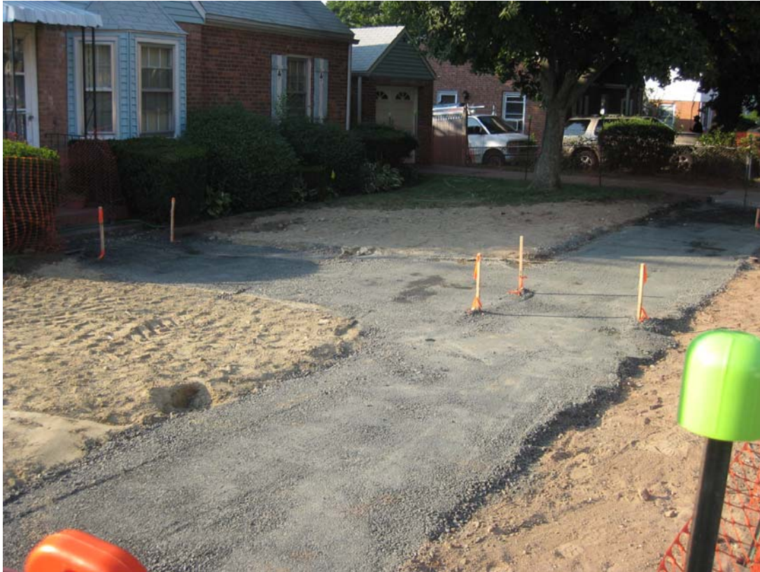
View looking northeast from Prospect Lane showing property backfilled and prepped for restoration.
