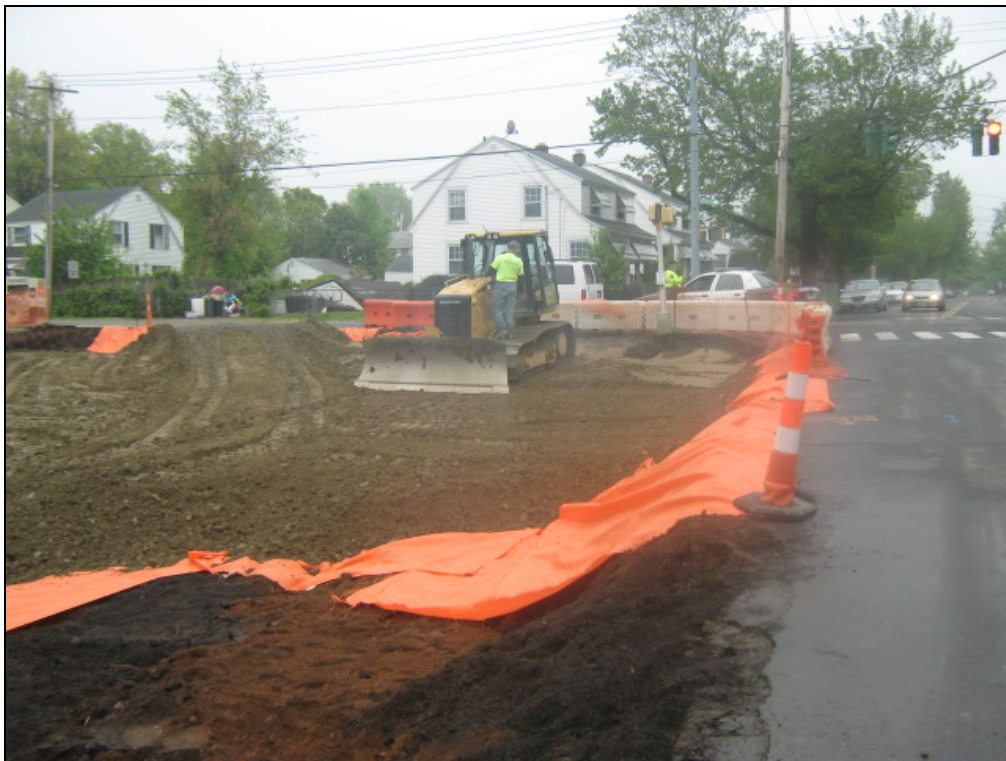
View looking south toward intersection of Morse and Newhall streets during placement of backfill material.
