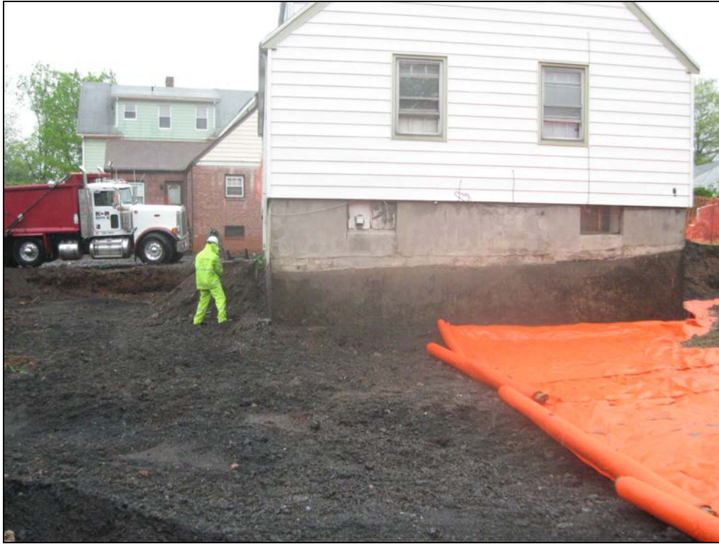
View looking east at excavated side yard with marker barrier being installed.
