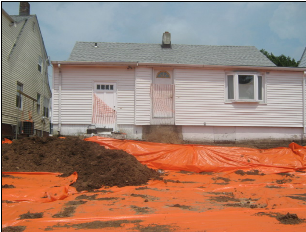
View looking north at excavated back yard following placement of marker barrier.
