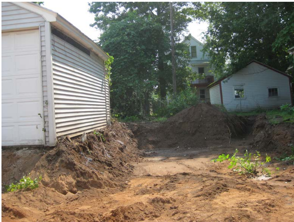
View looking East at excavated back yard and garage marked for concrete
