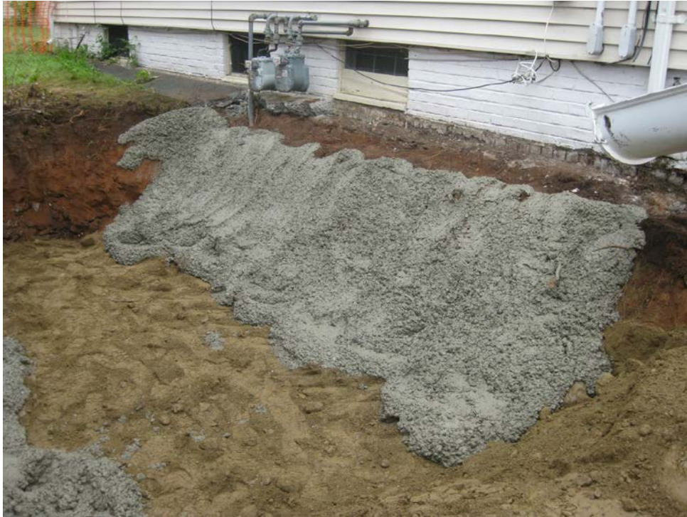
View looking south at extent of excavation adjacent to house during placement of concrete barrier
