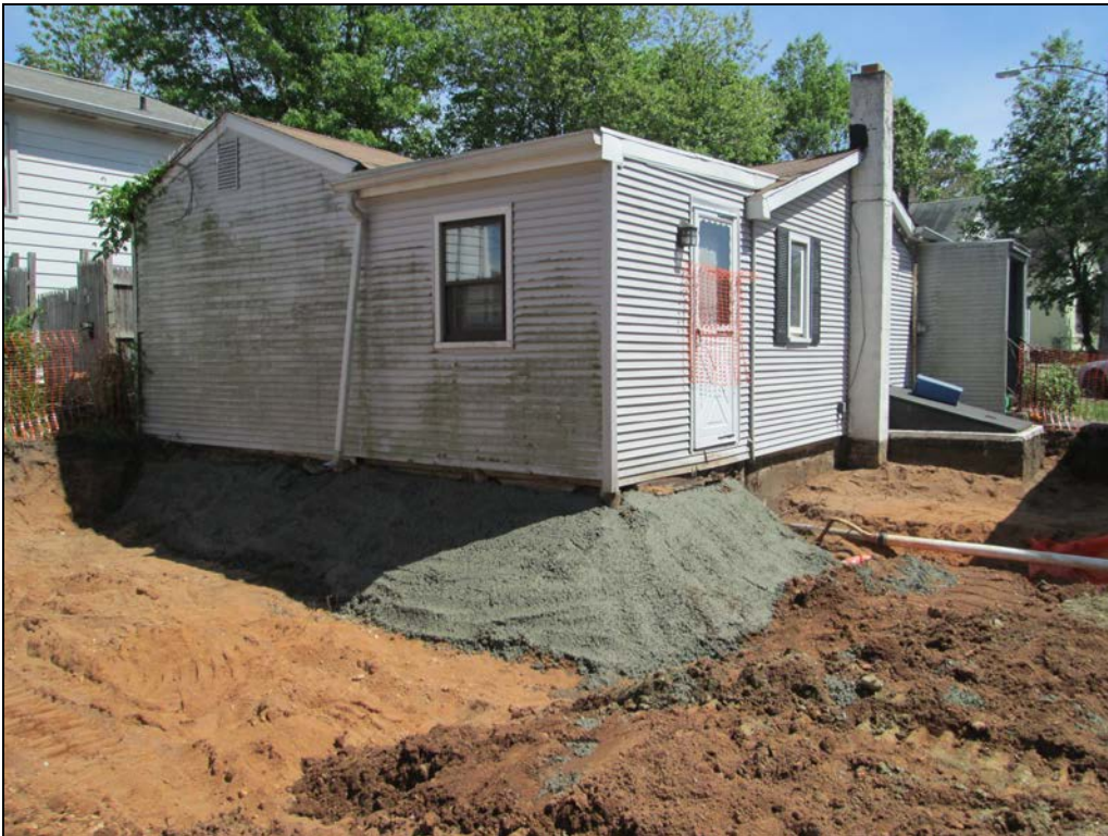
View looking southeast at excavated yard following placement of concrete marker barrier.
