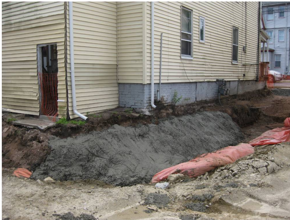
View looking Southeast at excavation along North side of house following placement of marker barrier
