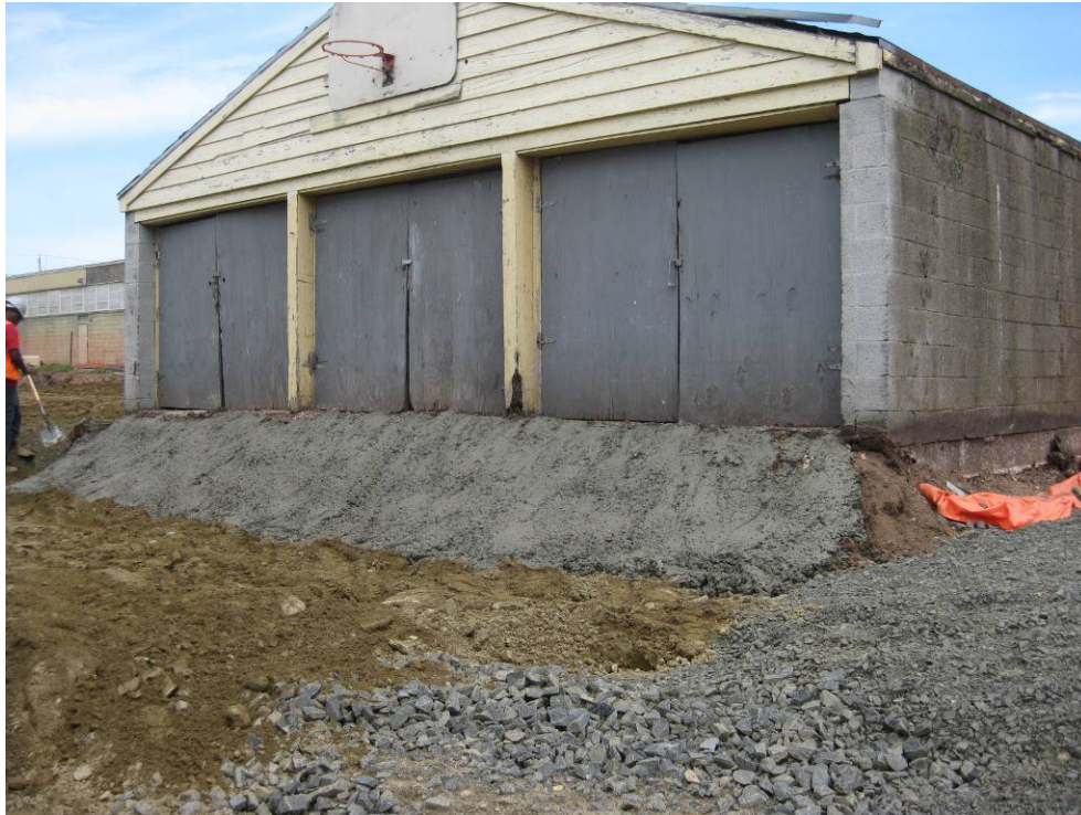
View looking Northwest at excavated in front of garage following placement of marker barrier
