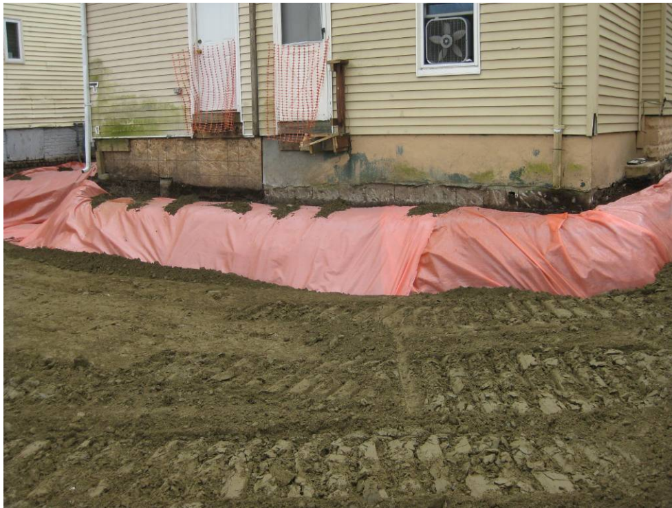
View looking Southeast at partially backfilled back of house following placement of marker barrier
