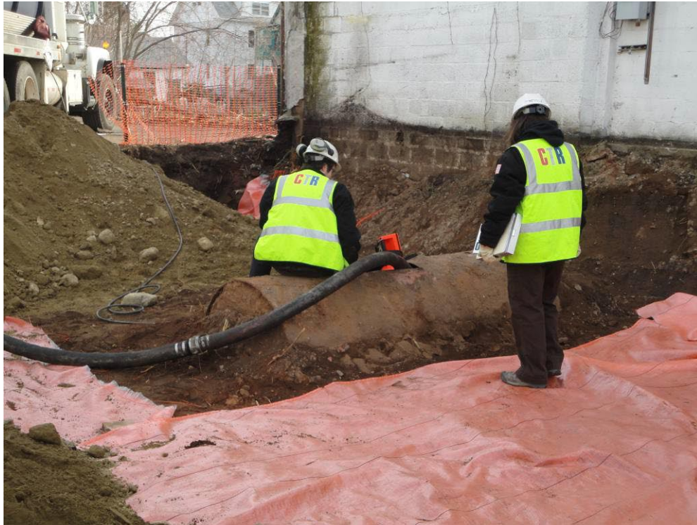
View looking northeast at abandoned UST identified behind the Church building
