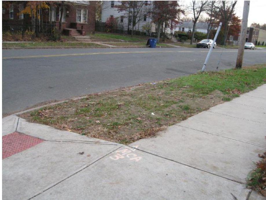
View looking Southwest at excavation area at the intersection of Morse Street and Shelton Avenue
