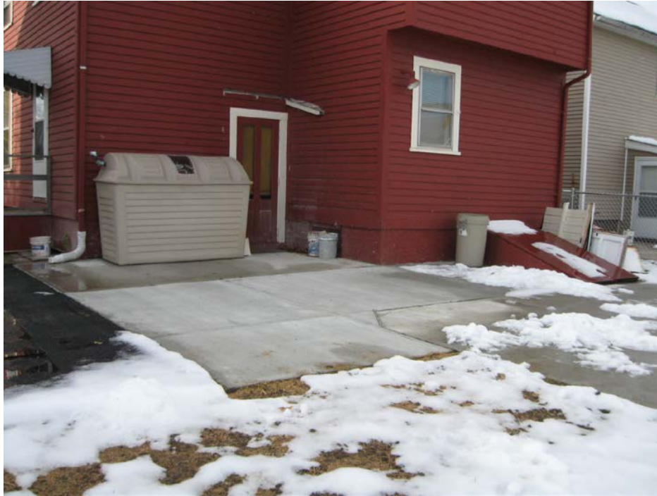
View looking Southeast at partially restored concrete pad and newly installed above ground storage tank
