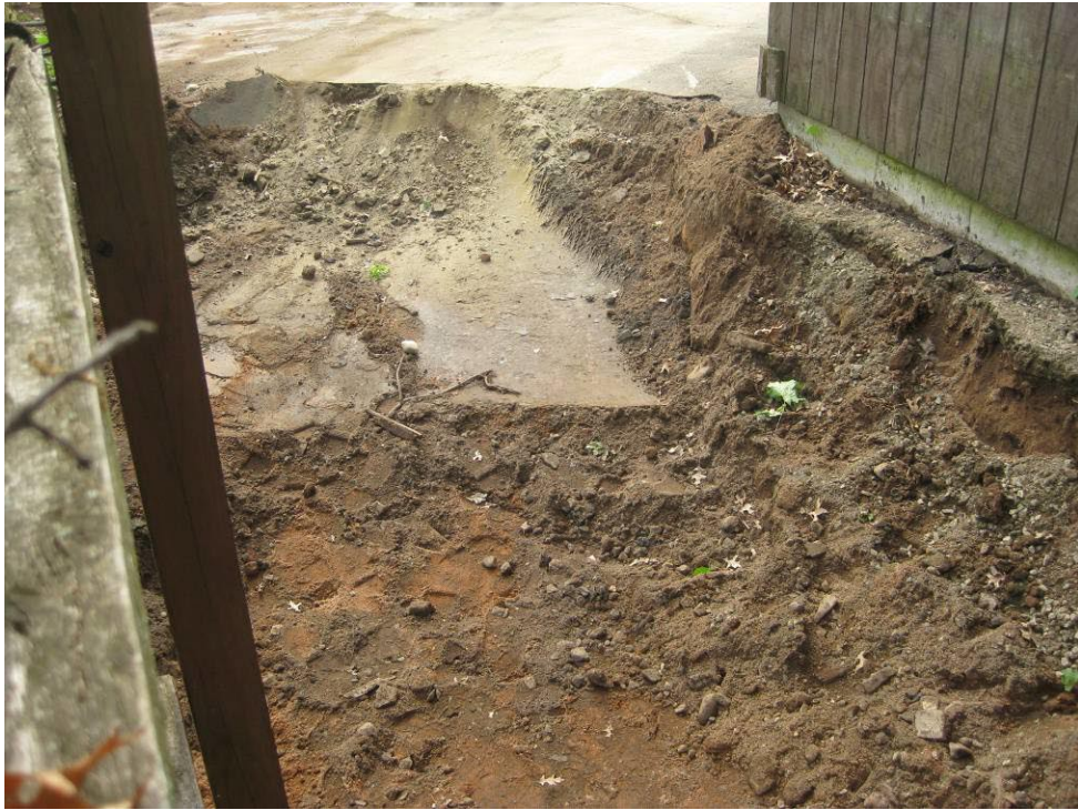
View looking East at excavation area between fence at 462 Shelton and garage at 293 Morse
