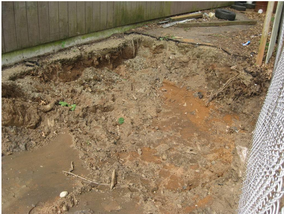
View looking Southwest at excavation area between fence at 462 Shelton and garage at 293 Morse
