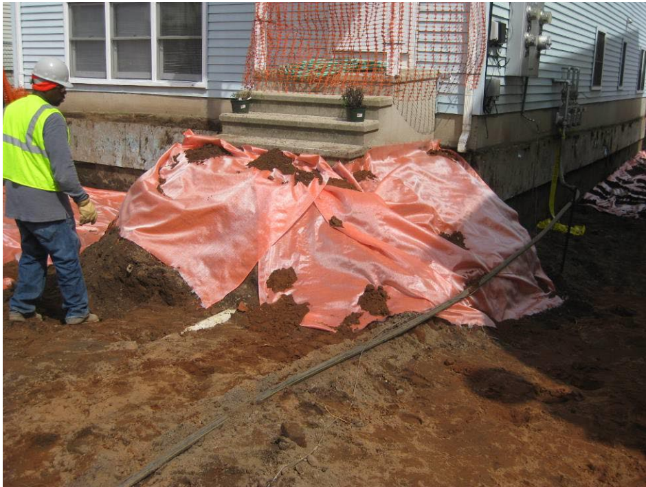
View looking Northeast at excavation area as marker barrier is placed around front entry
