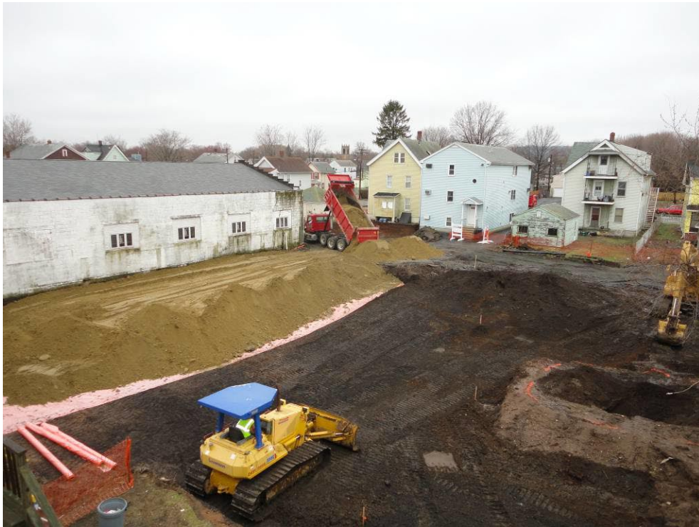
View looking Southwest at partially backfilled yard following placement of marker barrier
