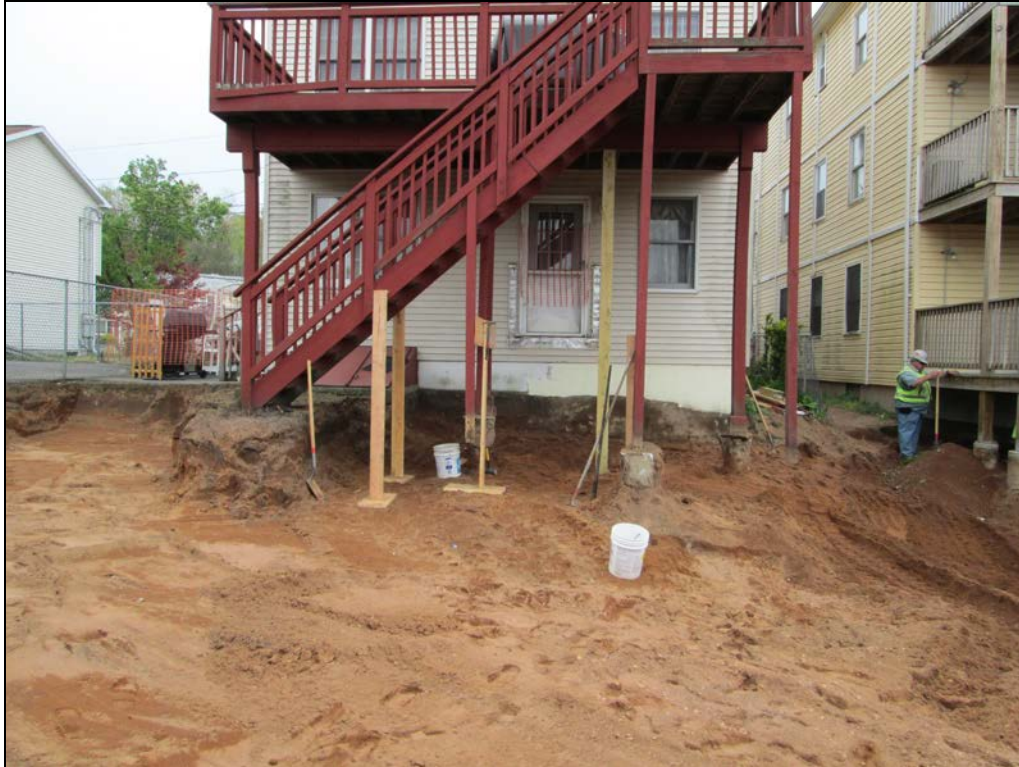
View looking south at excavated back yard. Deck was braced to allow excavation of fill beneath the footprint of the two-story deck.
