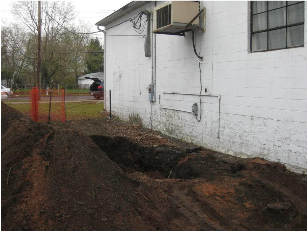
View looking East at area of UST removed as part of excavation activities
