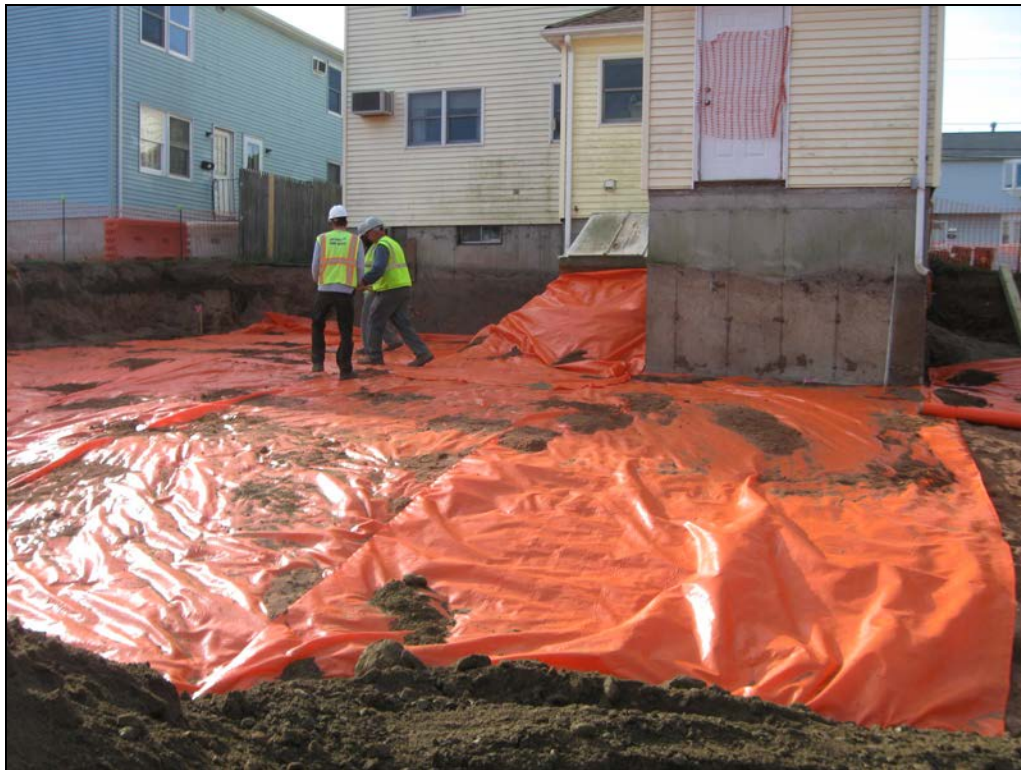
View looking south marker barrier being placed at base of excavation in back yard.
