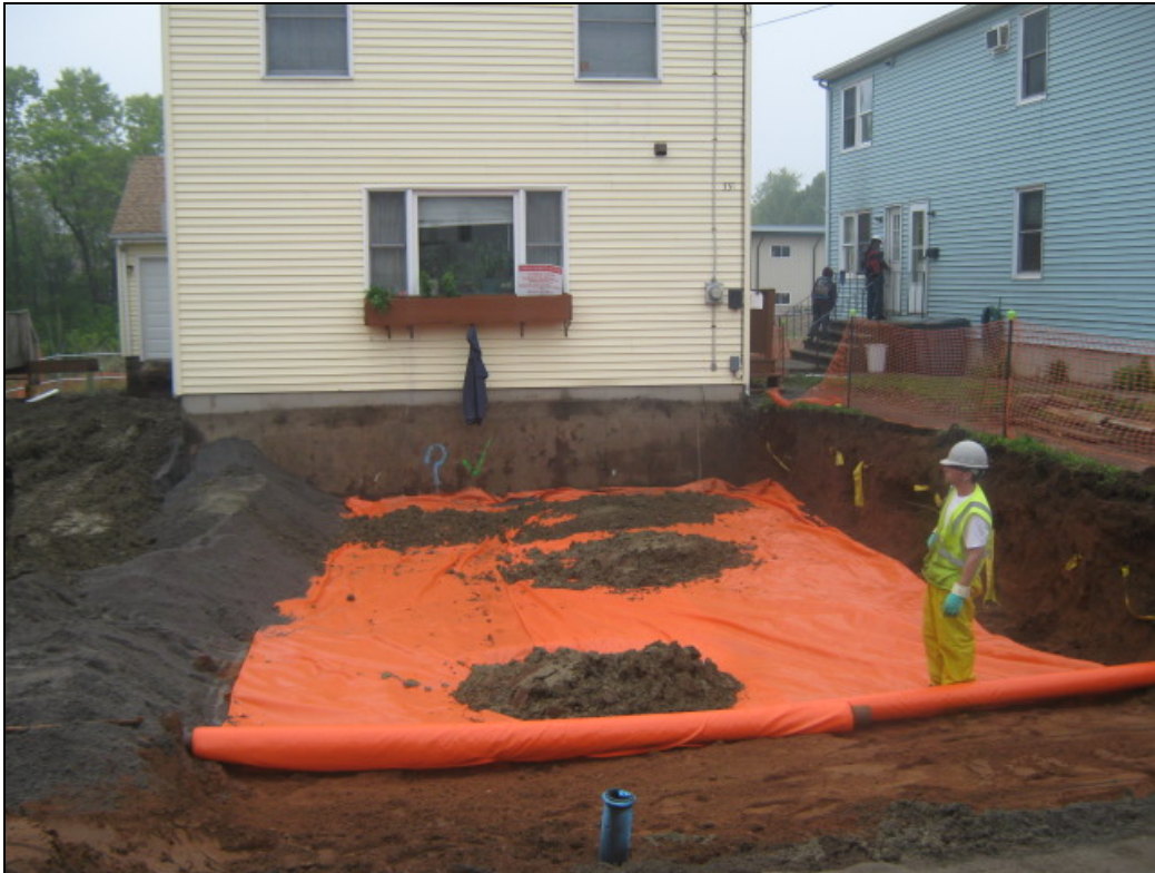
View looking north at marker barrier being placed at the base of excavation in front yard.
