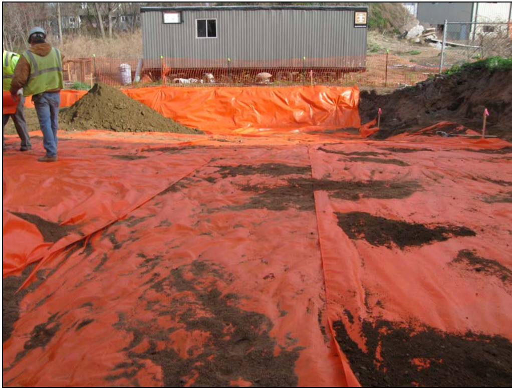
View looking north at marker barrier placed at base of excavation in back yard.
