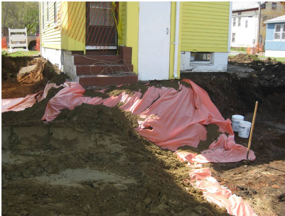
View looking West at excavation area at rear of house following placement of marker barrier
