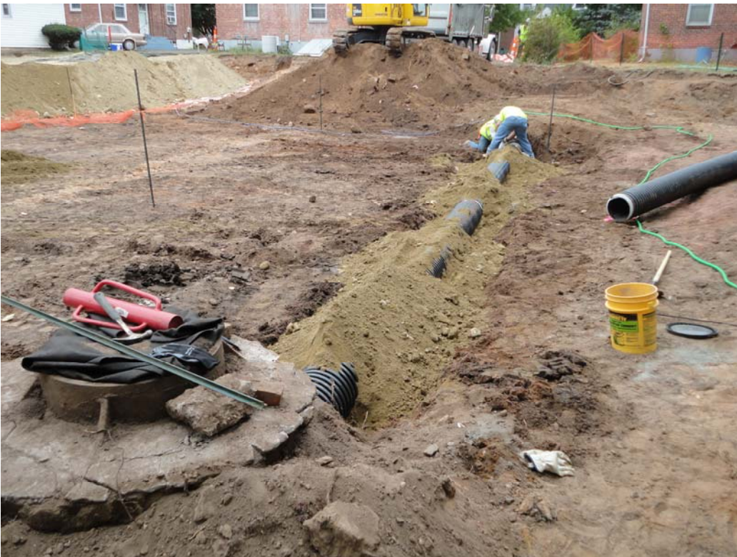
View looking southwest at repair of discharge line running from catch basin to storm sewer along North Sheffield St.
