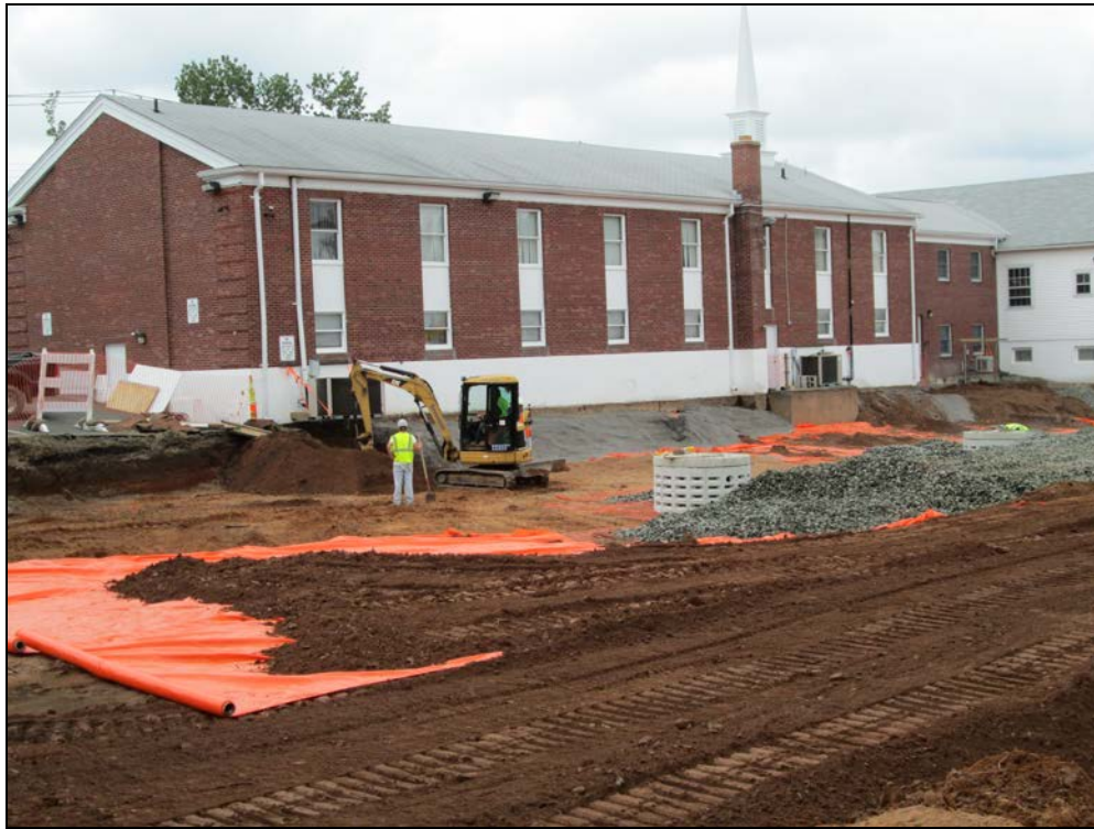
View looking northwest at back parking area during installation of drainage features and marker barrier.
