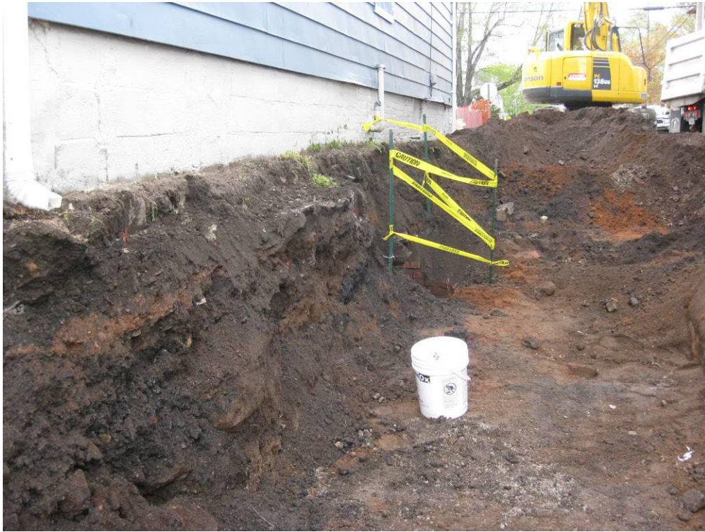
View looking West at existing drywell adjacent to north wall of foundation
