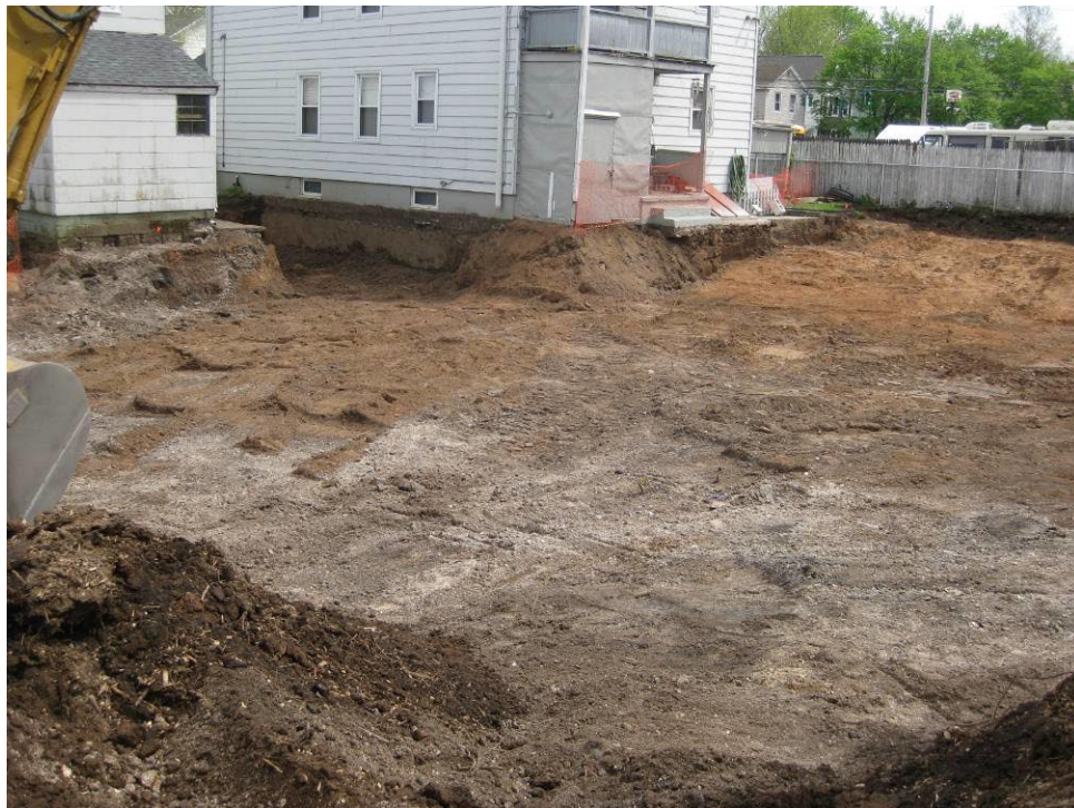
View looking Southeast at excavation area including soil wedge left in place around back stairs
