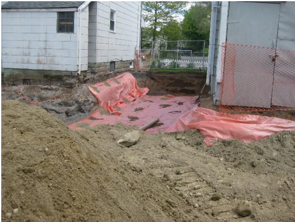
View looking East at excavated side yard to the South of the house following placement of marker barrier
