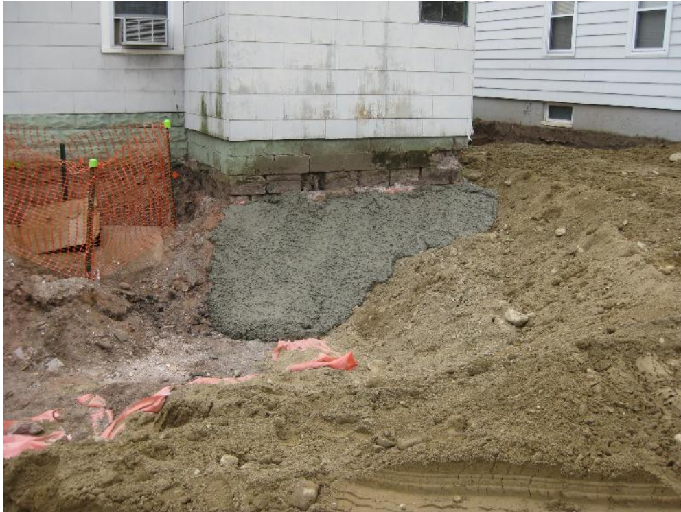
View looking East at excavated back yard following placement of marker barrier. In this photo, the area of the excavated UST is surrounded by orange construction fencing.
