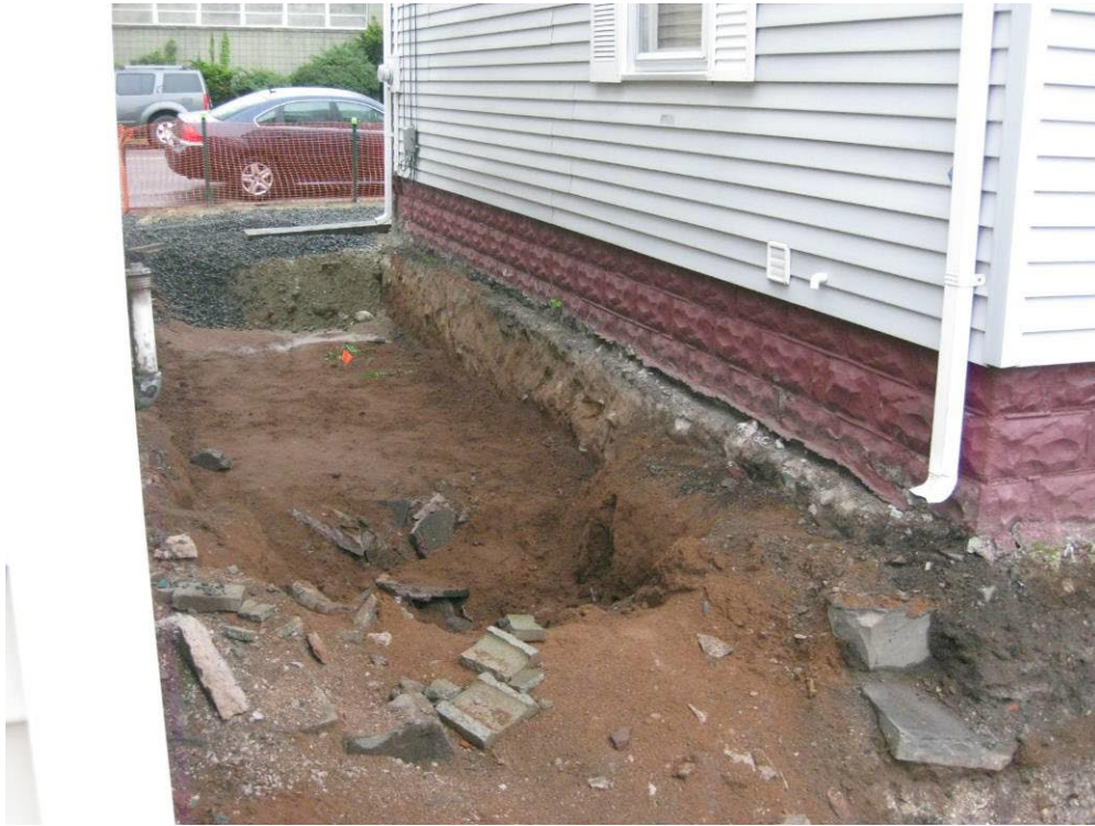
View looking East at excavated side yard to the North of the house
