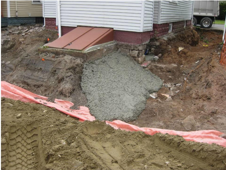
View looking East at excavation in back yard following placement of marker barrier around soil wedge left on west side of house and basement entrance
