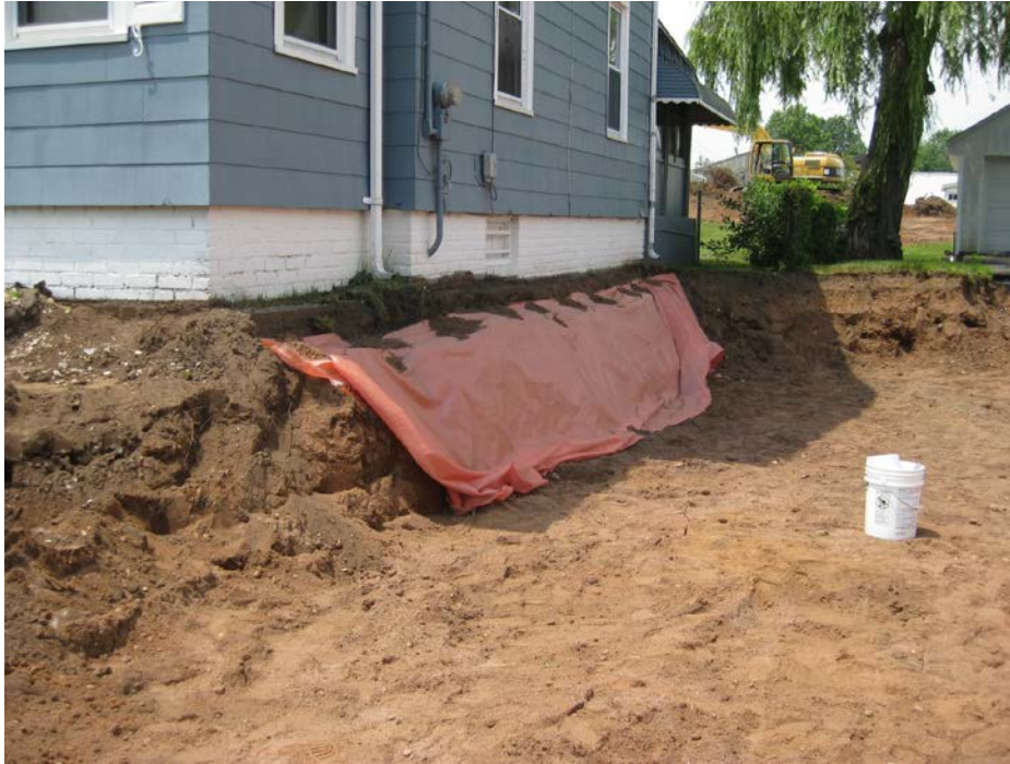
View looking West at excavated side yard following placement of marker barrier
