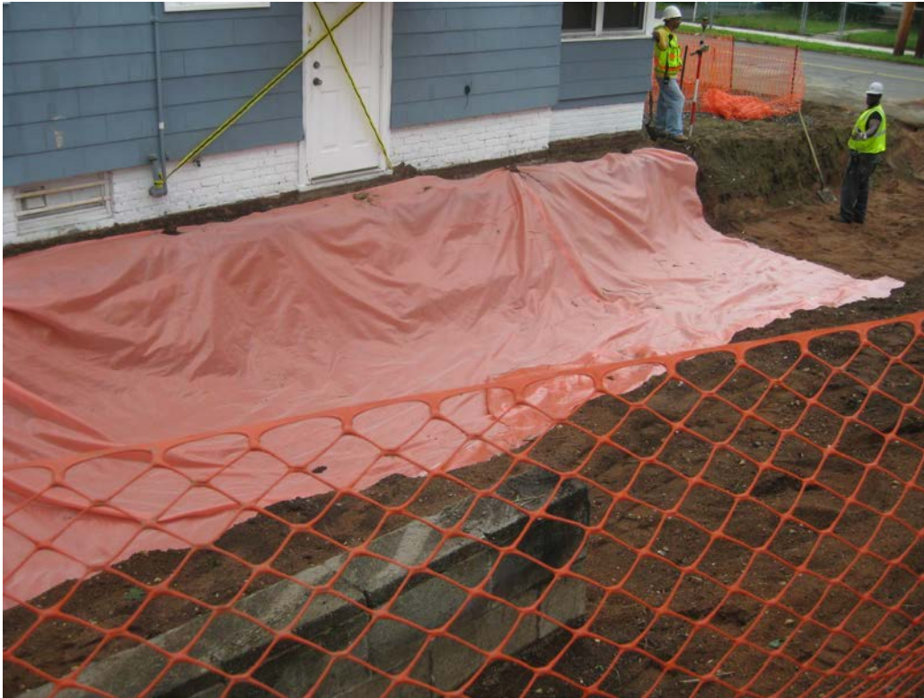
View looking Northeast at excavated side yard following placement of marker barrier
