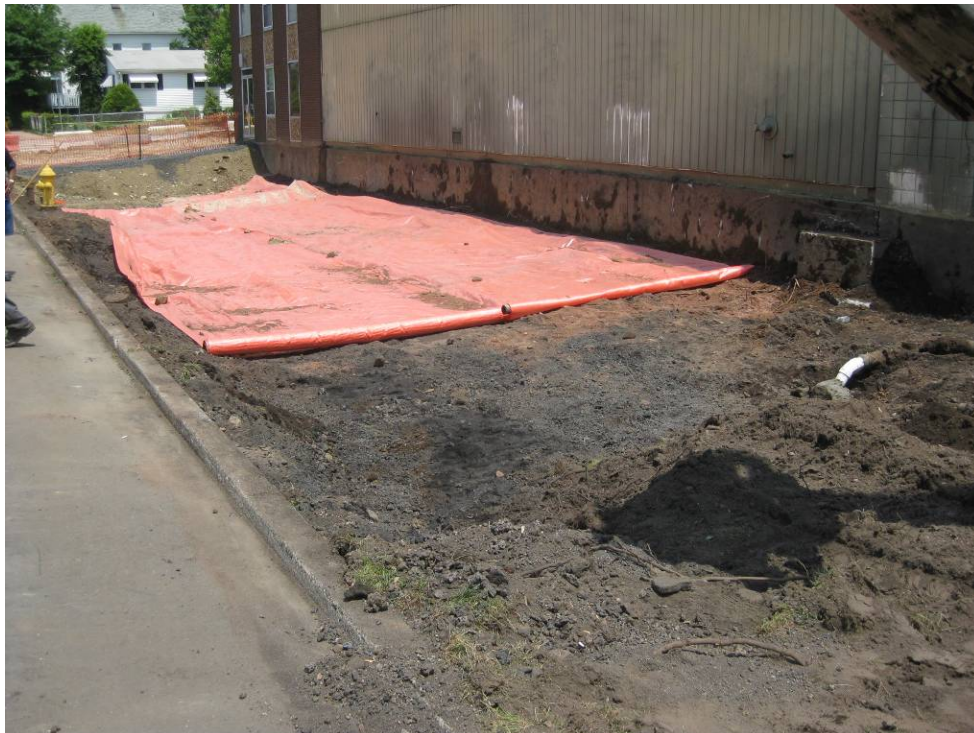
View looking Northwest at Southern side of building during placement of marker barrier
