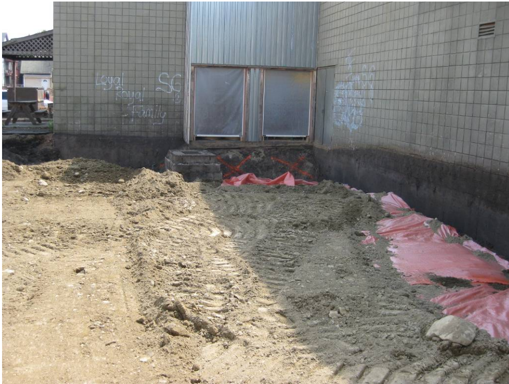
View looking South at partially backfilled area with marker barrier and sidewall marked out for concrete
