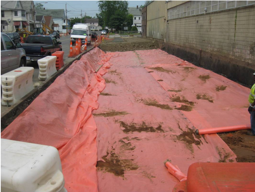
View looking North at excavated Western side of property during placement of marker barrier
