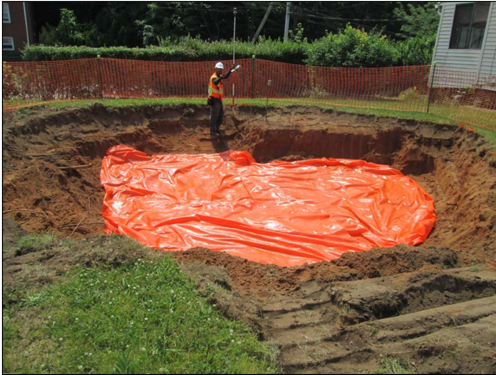
View looking east at excavation in side yard during placement of marker barrier.
