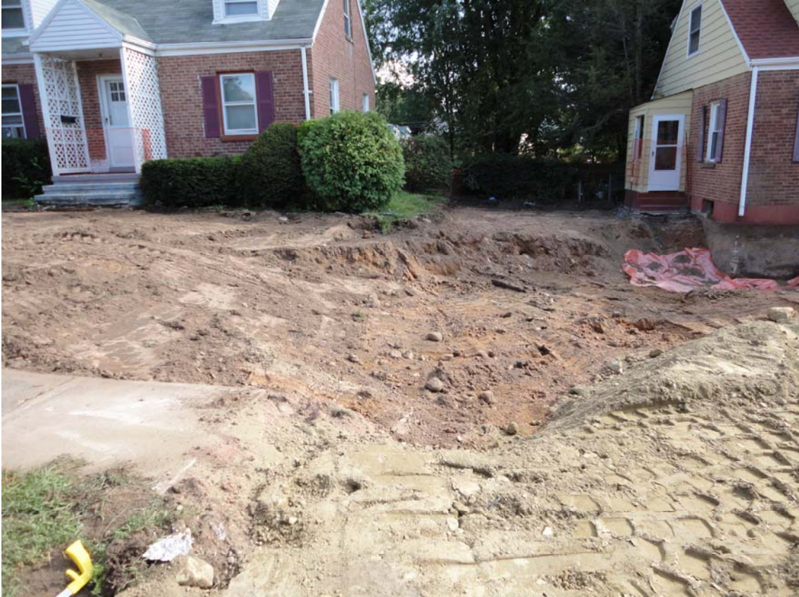
View looking south at excavation in front yard between 92 Morse Street and adjacent property.
