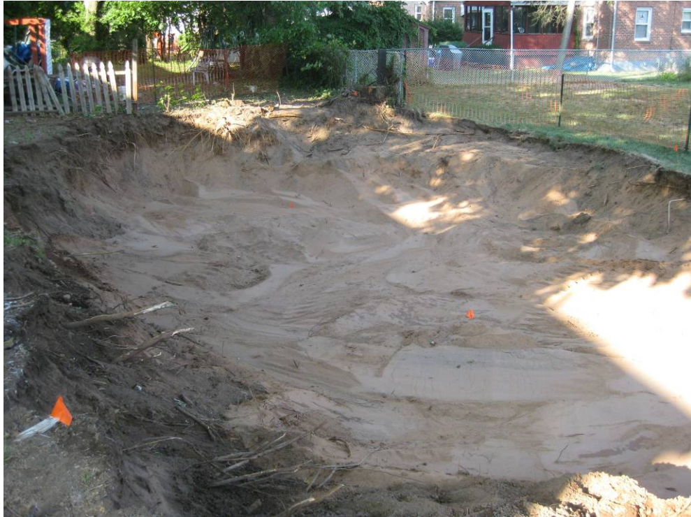
View looking north at extent of excavation in backyard of 957-959 Winchester Avenue.
