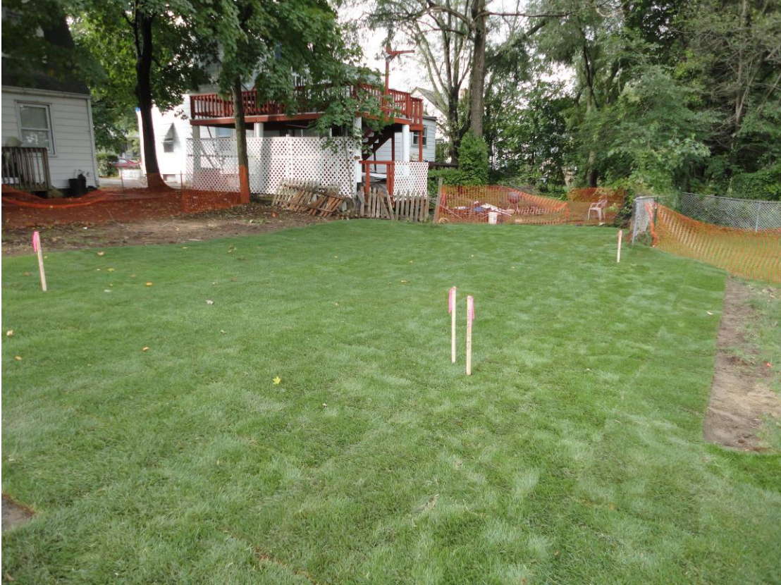
View looking northeast at partially restored backyard prior to installation of fencing.
