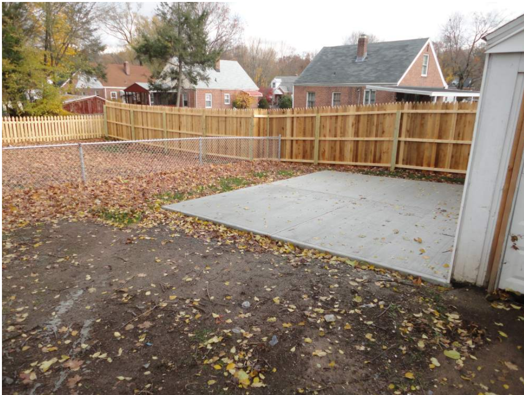
View looking southeast at restored backyard including newly installed fencing and concrete pad.
