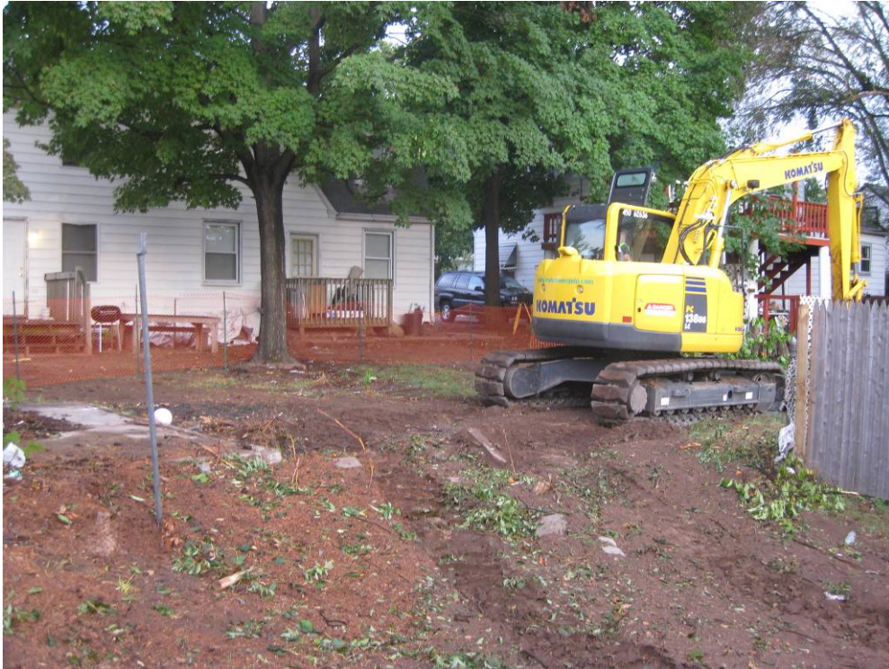
View looking northwest from backyard of 10 North Sheffield Street at excavation activities beginning at 957-959 Winchester Avenue.
