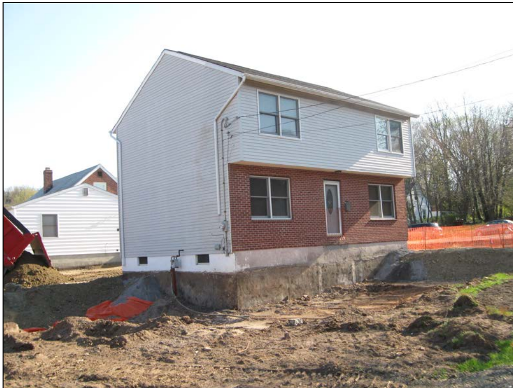
View looking northeast at excavated front yard prior to marker barrier being installed.
