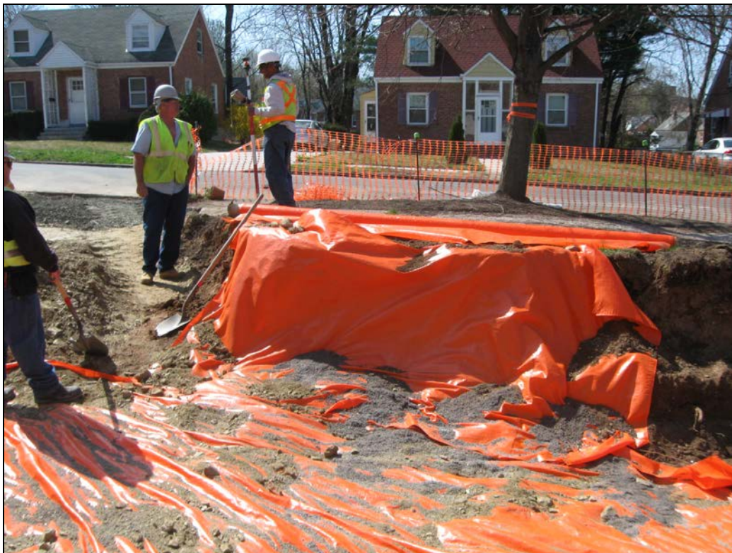
View looking south at marker barrier being installed around perimeter of tree that was retained in accordance with the Tree Sampling Plan.
