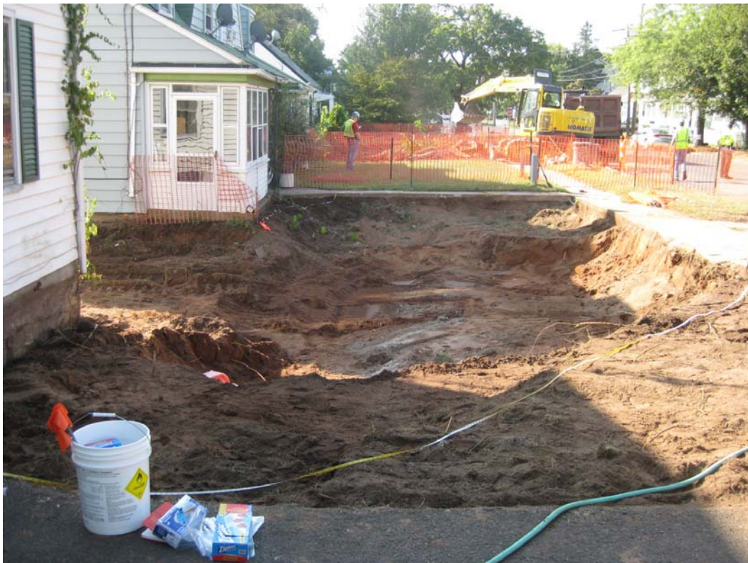
View looking south at excavation continuing across front yards of 979-981 and 985 Winchester Avenue.
