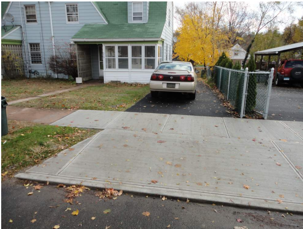
View looking east at newly installed driveway along south boundary of 979-981 Winchester Avenue.
