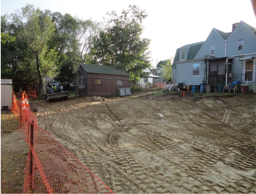
View looking southwest at backyard of 979-981 Winchester Avenue following placement of backfill.
