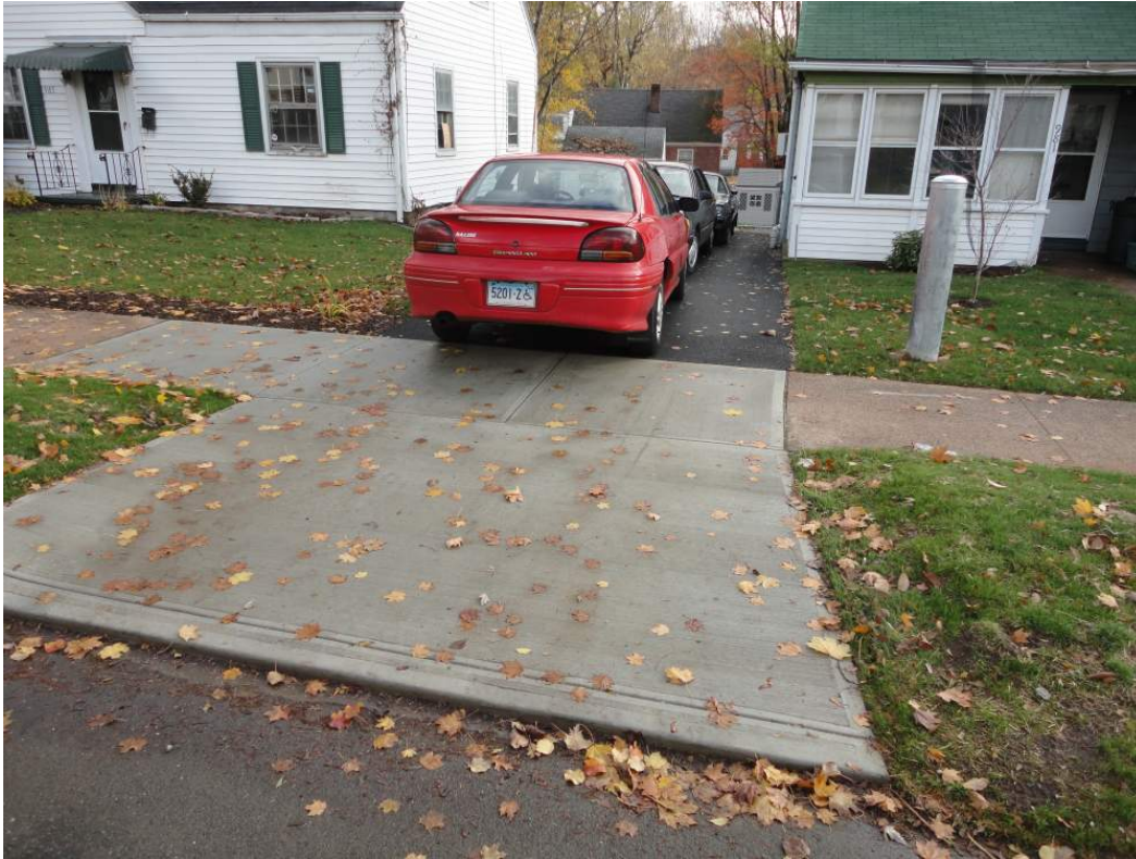
View looking east at newly installed driveway along north boundary of 979-981 Winchester Avenue.
