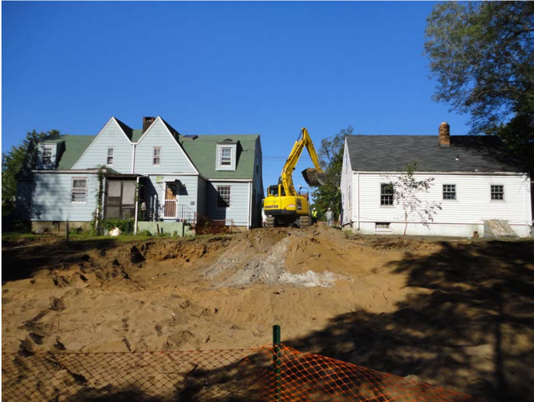
View looking west at extent of excavation in back yards of 979-981 and 985 Winchester Avenue.
